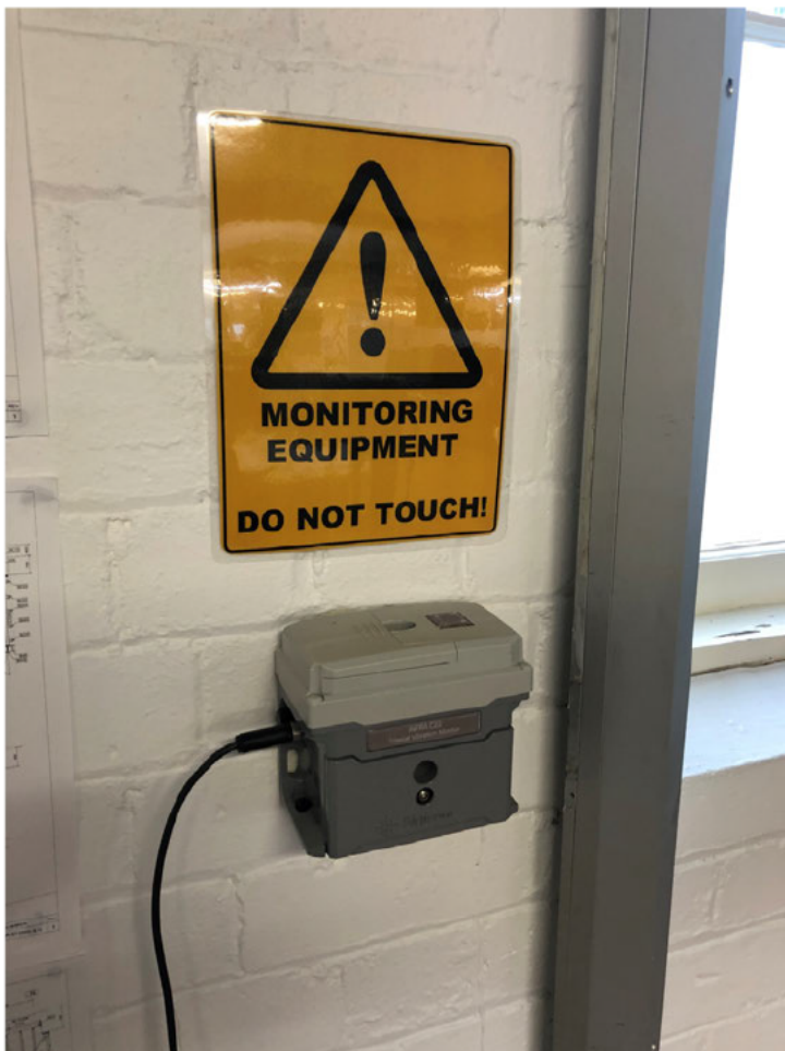
Figure 3 – On site real-time vibration monitor at 25 Hickson Road
