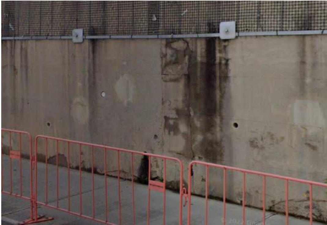
Figure 7: Cracking at the location of SBR 3.2.
