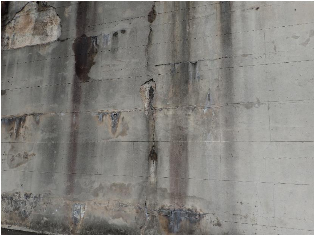
Figure 8: Cracks in the render at the location of SBR 3.3 (prior to the installation of the protective mesh).
