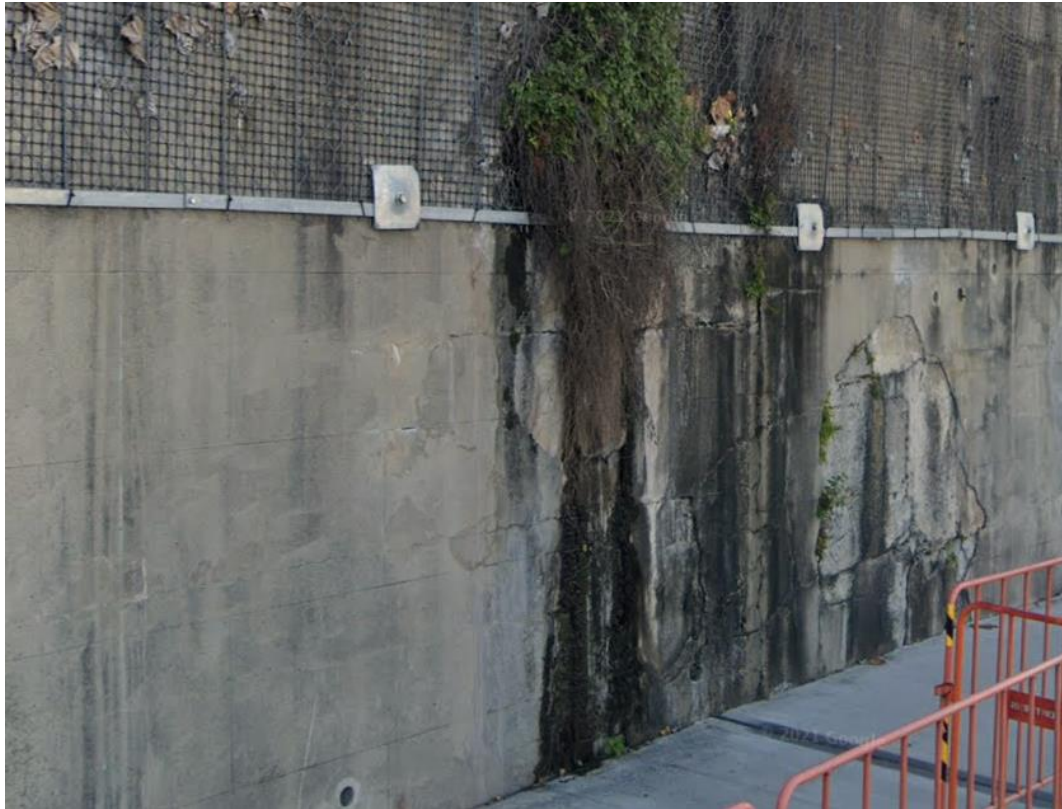
Figure 9: Cracking and intrusive vegetation at the location of SBR 3.4.
